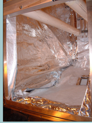
Keeping the insulating vacuum separate from the cavity vacuum permits the use of multilayer insulation (MLI). Reduced heat load on the LN2-cooled thermal shield saves nitrogen and allows a thinner, conductive shield. Prefabricated copper panels hang from two rectangular LN2 manifolds mounted to the top of the box, standing off of the interior with G10 buttons.
