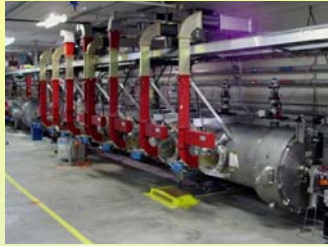
Cryomodule installed in FEL
