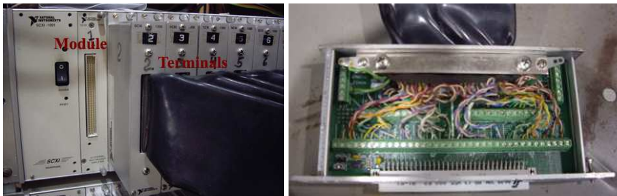
FIG. 5: Left to right: terminals connected to modules, with one disconnected; terminal box with lid removed
